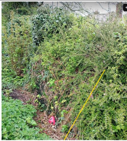
Note the angle of the fence post which is leaning down the bank.
